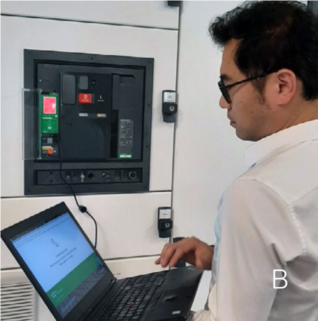
Figure 1 A. Direct connection with MasterPact MTZ only B. Connection through Service Interface for ComPact / PowerPact equipped with MicroLogic control unit, MasterPact NT/NW
