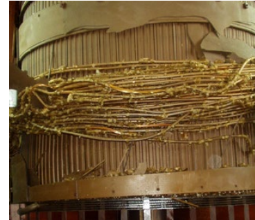
Collapsed tap winding
