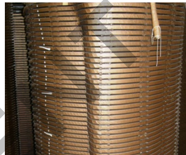
Buckling of winding
