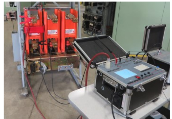
MAC-TS4 Vacuum Bottle Test Set testing vacuum interrupters installed in GE PowerVac circuit breaker without disassembling the breaker
