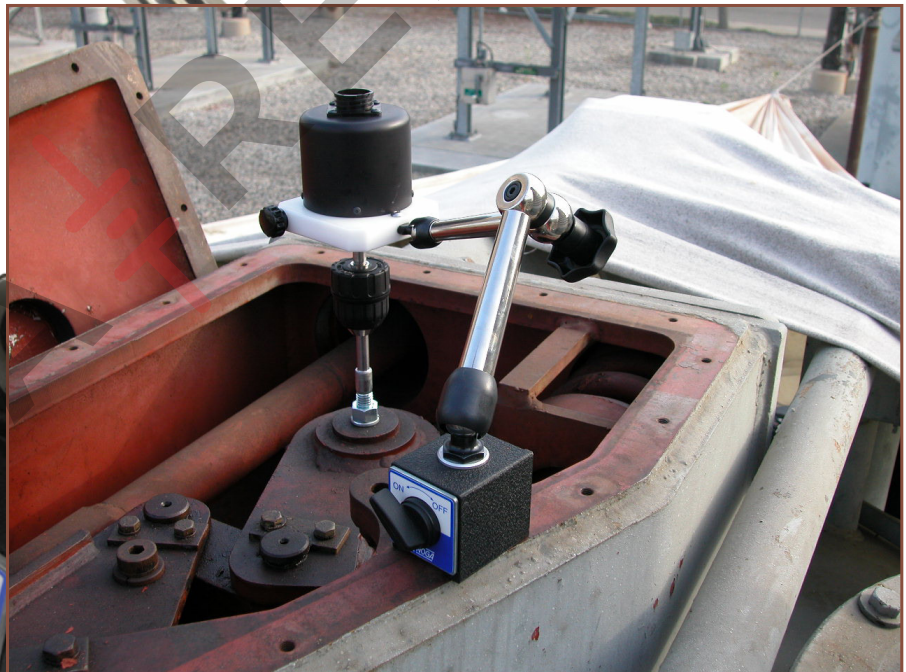
Type 3 rotary transducer on a Federal Pacific breaker
