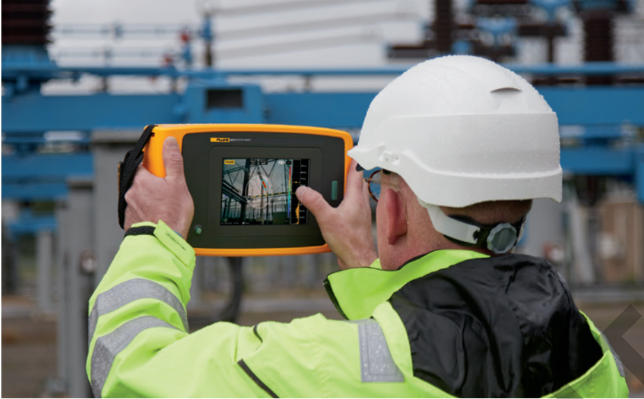
Image taken of the ii910 Precision Acoustic Imager detecting partial discharge in a high voltage application.
